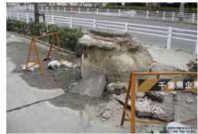
Manhole that rose due to liquefaction (2011 Great East Japan Earthquake)
