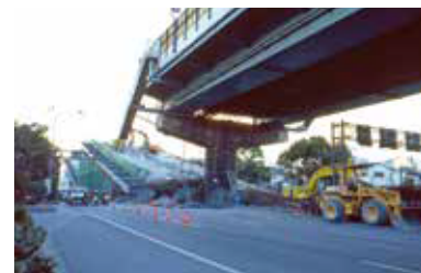
Collapsed Hanshin Expressway
